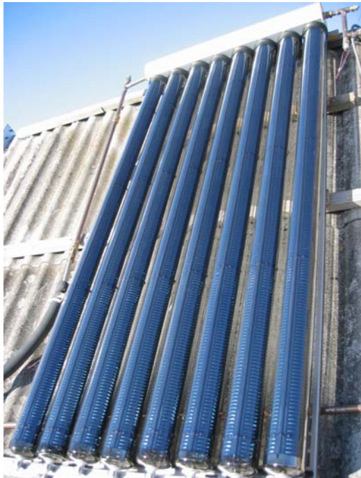
Figure 1. SEIDO5-8 on the roof of the lab at DTU
